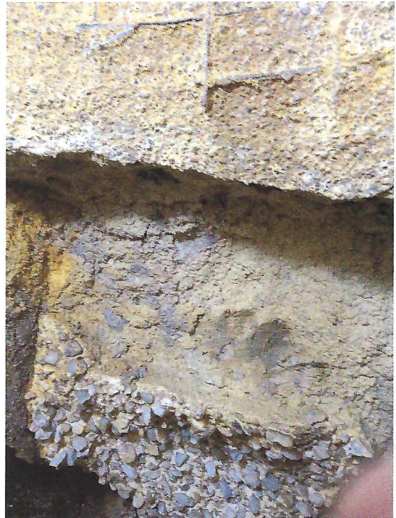
Manhole #2: Fully Eroded Side Wall with Exposed Dirt. Remaining Concrete has Exposed Rebar.
