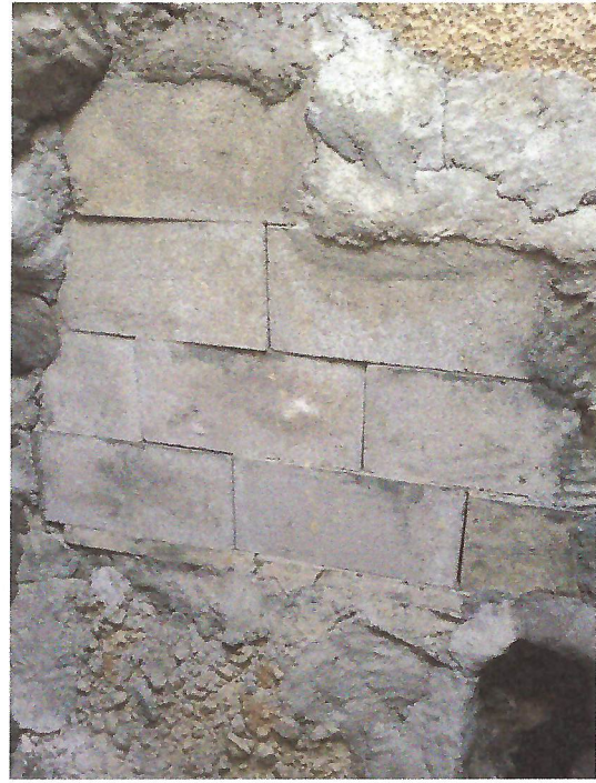
Manhole #2: Rebuilt Side Wall with Concrete Blocks to Fill in Voids and Restore Structural Integrity
