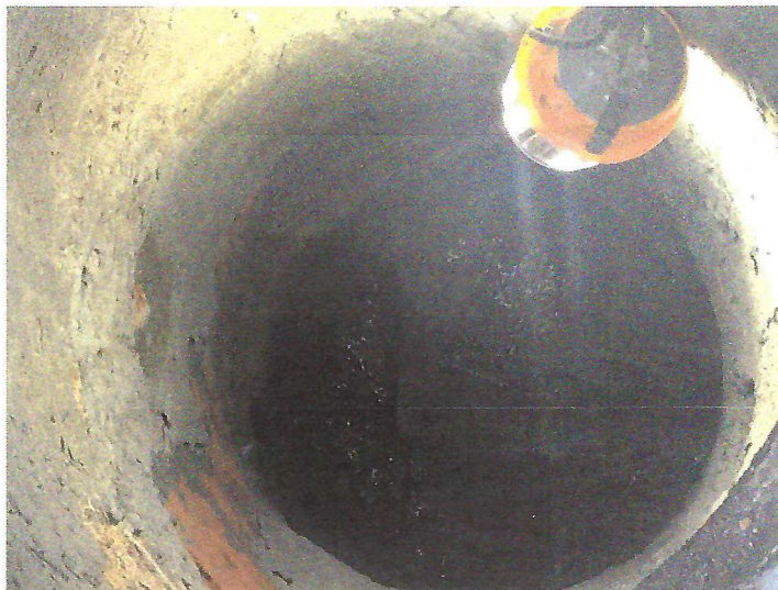
Manhole #1: Existing Deteriorated Condition
