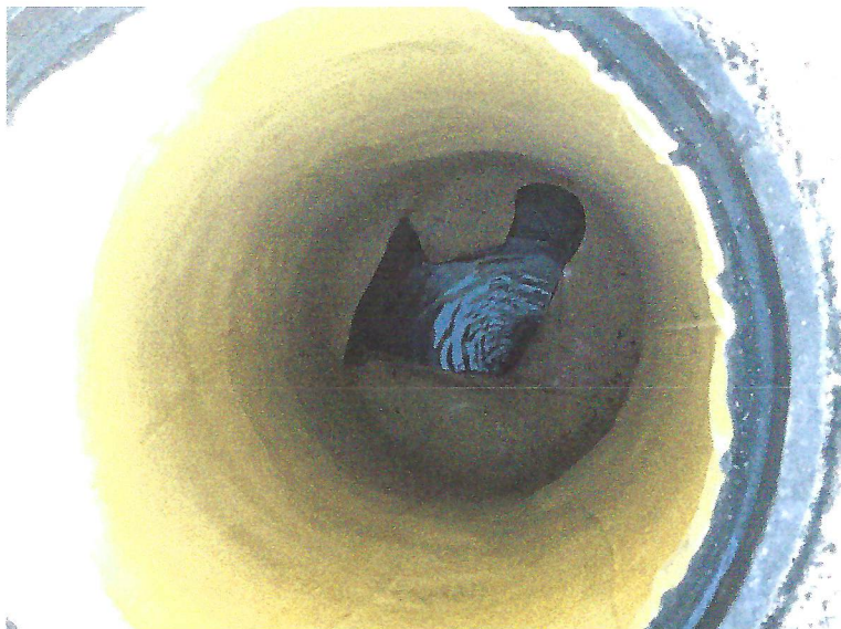
Manhole #1: Completed Rehabilitation. The New Cured-in-Place Liner will Prevent Future Concrete Erosion
