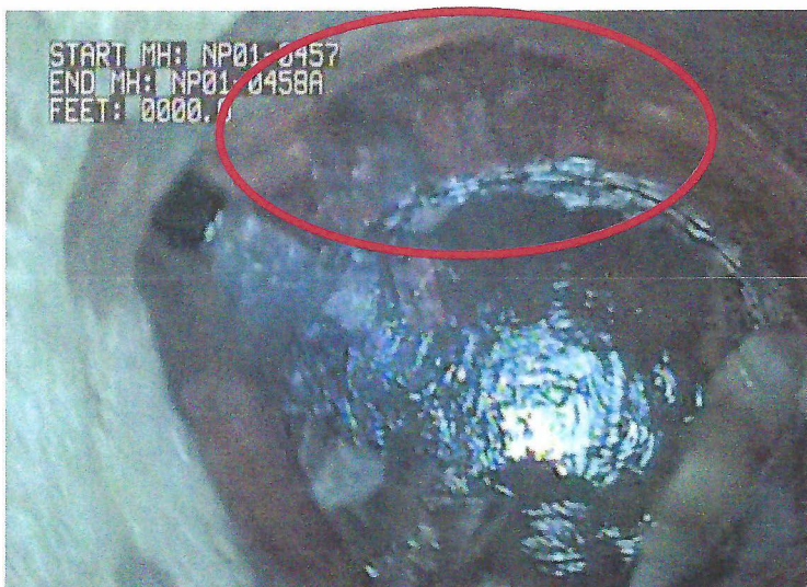
Manhole #1: Existing Hole in Back Wall
