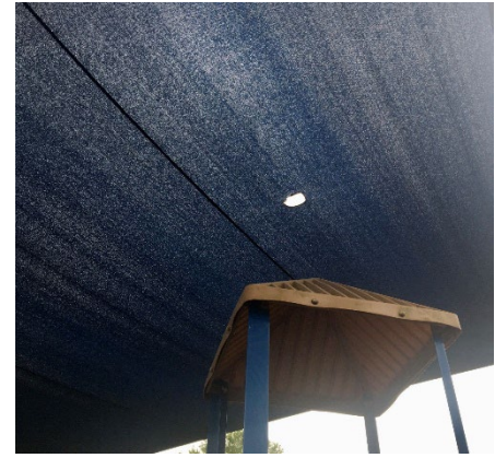
Damage to the Port O Call Park Shade
