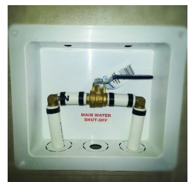
Example of the House valves in a garage
