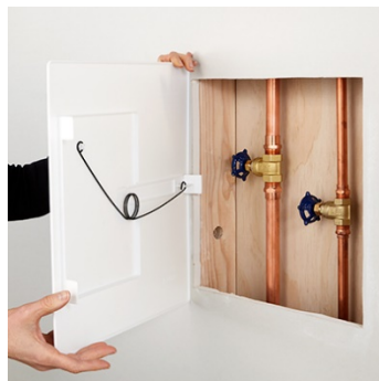
Example of the House valves inside a closet
