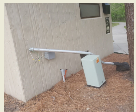
Damage to the security light at Flying Bridge park
