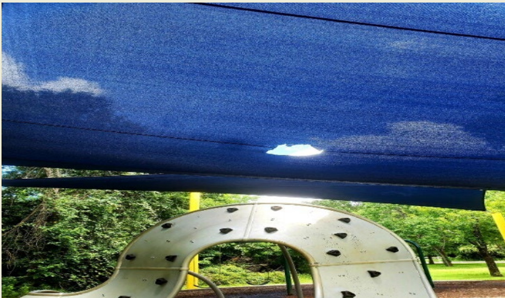
Newly installed park shade at Flying Bridge Park damaged
